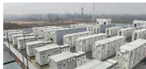
Hubei Gaoqiao 50MW/100MWh Energy Storage Project SC(B)-3450/10kV Cast Resin Dry Type Transformer
